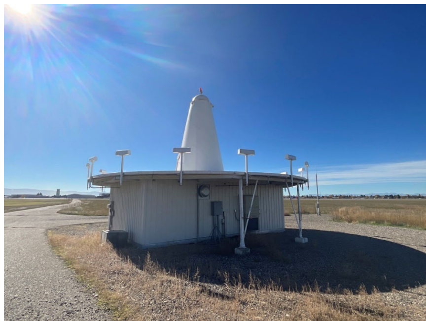
Figure 6.17. VOR at BZN, view to the south.
