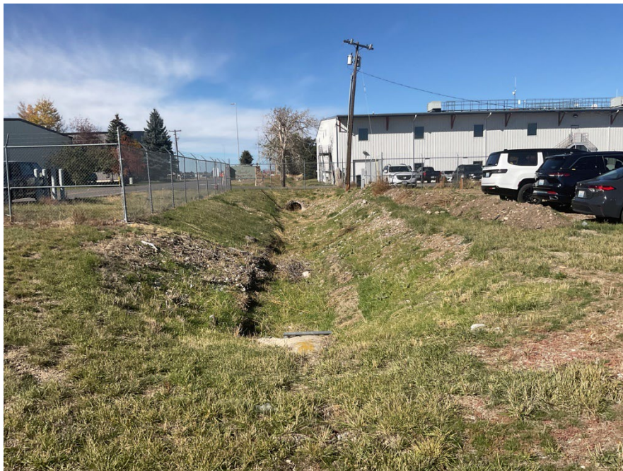
Figure 6. 24GA0743 abandoned segment at Taxiway "H," view to the east.
